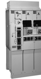
Old compact switchgear
